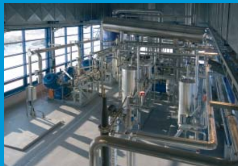
Woikoski carbon dioxide handling plant started up in spring 2006.
