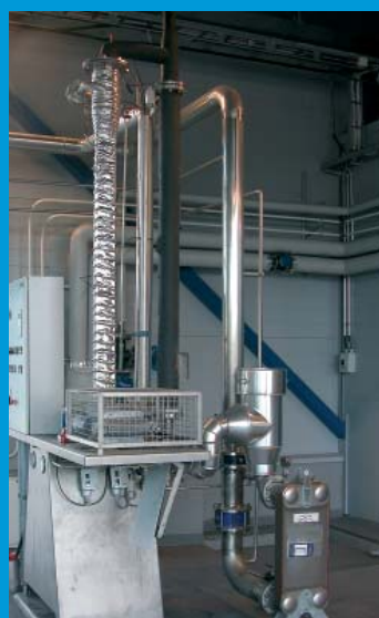
The carbon dioxide handling plant produces also dry ice.
